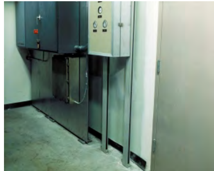
Figure 157: Two different ways to support control panels: using a metal plate attached to floor and ceiling with steel angles (left); using struts extending to floor and ceiling (right).
