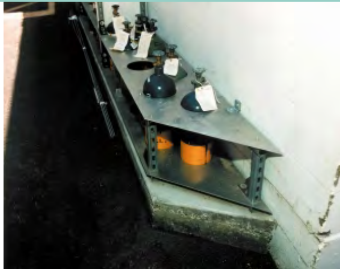
Figure 82: Small gas cylinder storage.
